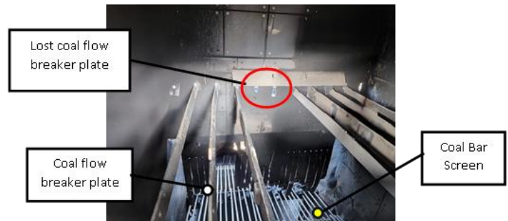
Fig. 1. The coal flow breaker plate on the vibrating screen component is damaged.
