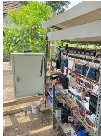
Fig. 1. Realization of solar power generation for lighting loads.
