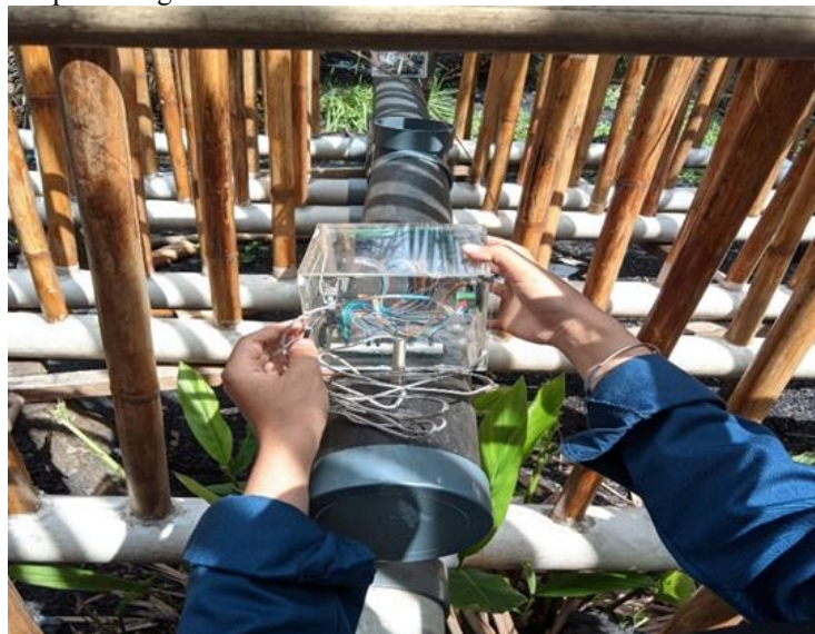
Fig. 4. Field installation of the dual-sensor thermocouple monitoring system on the PVC smoke pipeline.
