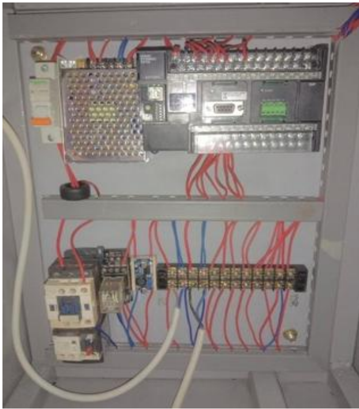
Fig. 6. Power and control system panel
