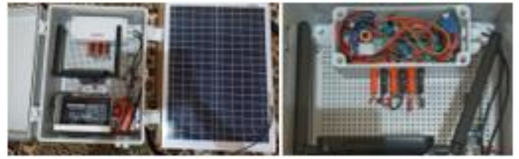
Fig. 6. Solar panel monitoring system.
