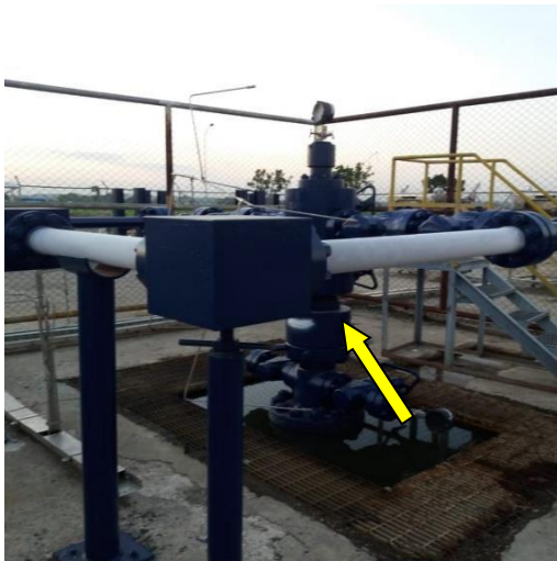
Fig. 2. The phenomenon of icing on valve wings in one of the gas field wells
