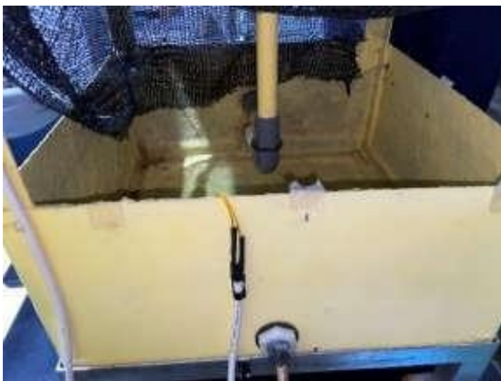
Fig. 5. Water basin Cooling Tower
