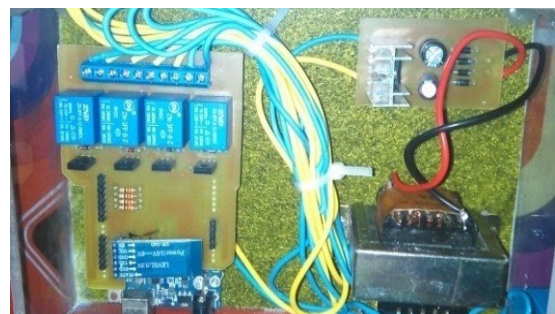
Gambar 13. Hardware control lamp system
