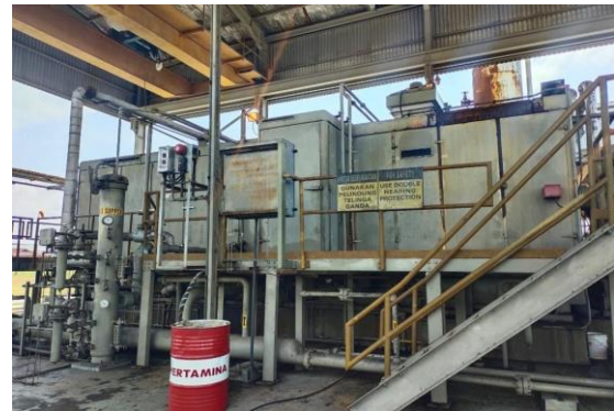
Gbr. 6 GE Turbin Gas PT.Pema Global Energi Tampak Samping
