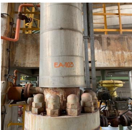
Gbr 1. Ammonia Preheater (62- EA-103)
