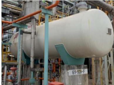
Gbr. 1 Refrigerant receiver (61-109-F)
