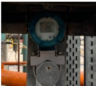
Gbr. 2 Level Transmitter
