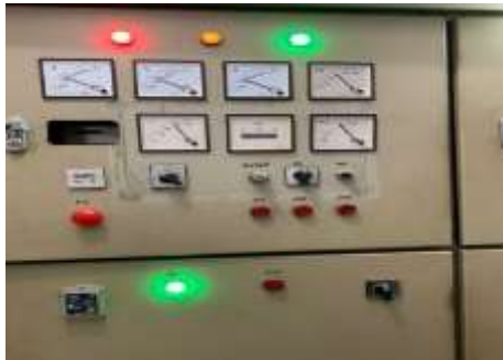
Gbr 4. Control Panel
