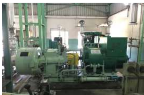
Gbr 3. Turbin Generator
