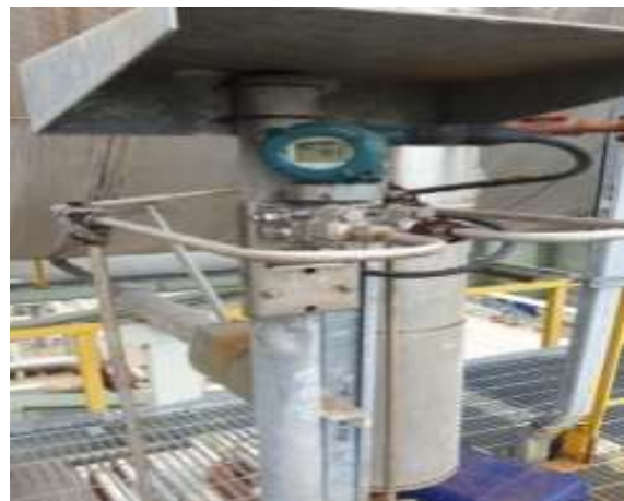
Gbr 2. DP Transmitter (61-LT-1030)
