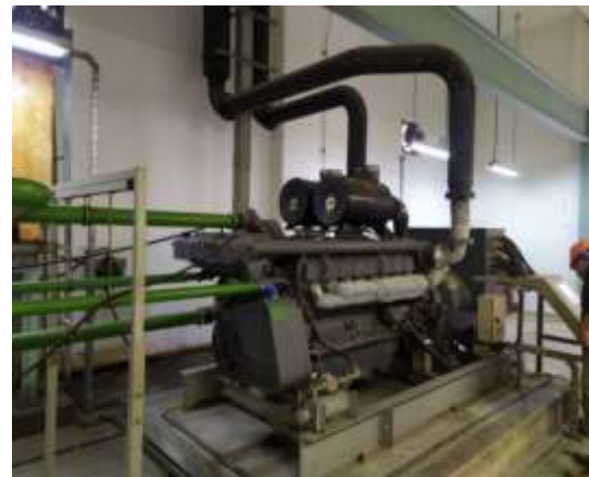
Gbr 2. Diesel Engine Generator 760 KW
