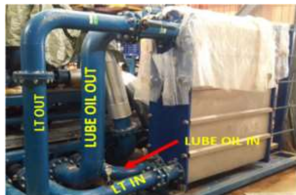
Gbr 4. Heat Exchanger (HE)
