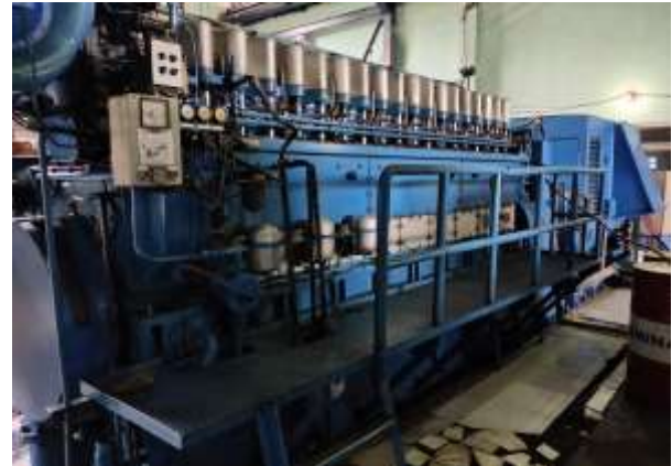
Gbr 8. Generator (PLTD) Tapak Tuan
