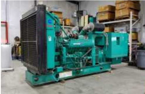
Gbr 1. Generator mesin diesel
