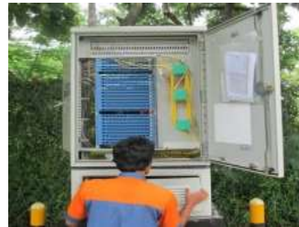
Gbr 3. Optical Distribution Cabinet
