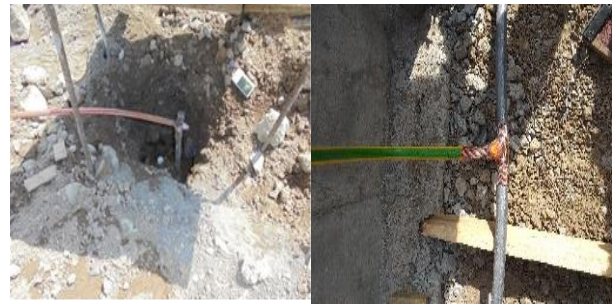
Gambar 10. Instalasi Grounding Root
